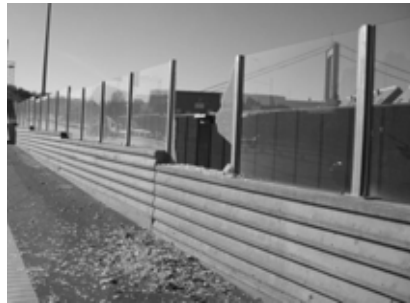
Figure 1.1 Damaged noise barrier along road E6 in the city of Gothenburg in Sweden
